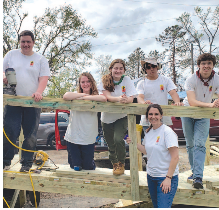
Building a wheelchair ramp was one of the several projects a team of students from Irving, Texas, completed on their spring break while helping with hurricane recovery in the Diocese of Lake Charles.
