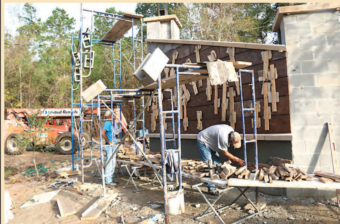
The success of the Return to the Lord campaign can be seen as the work continues on the entry gate to Camp Karol of Saint Charles Center in Moss Bluff. In photo 1, forms were built and readied for the pouring of concrete in late December. In photo 2, the work continued to the point where each side of the gateway were constructed and, as seen on the right entryway, bricks begin to adorn the bottom portion. In photo 3, workers continued placing the bricks, here on the backside of the left entryway. Preliminary plans are being discussed for the future construction of the main building at Camp Karol, to be named The Lodge.
