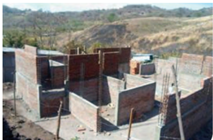
One of the projects on the agenda for the missionaries on this summer's trip is the completion of a rectory begun last year. Msgr. Daniel Torres said he was surprised at the progress from the photo as when last there, "we began by digging a ditch."
