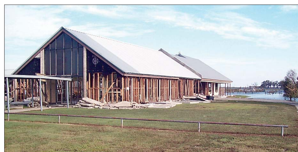
Our Lady of the Assumption Church in Johnson Bayou is merely a roof and the supporting two-by-fours following the more than 11-foot storm surge of Hurricane Ike.
