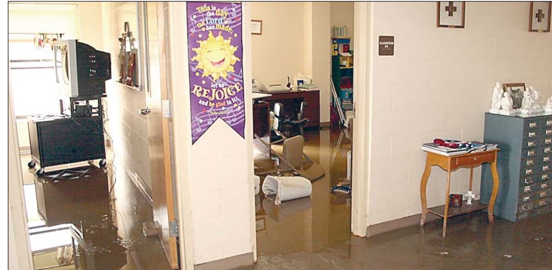
More than two feet of water damaged classrooms and furnishings in the Religious Education building at St. Peter the Apostle.
