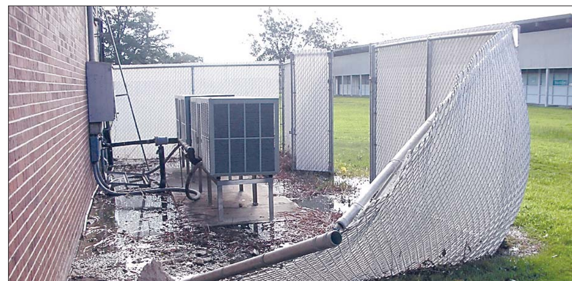
More than 30 inches of water inundated St. Mary of the Lake's buildings. Here even raising the outside air conditioning units didn't keep the deluge from damaging the units.
