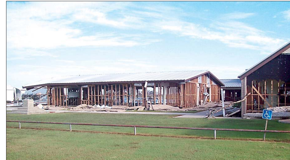
The hall and religious education building at Our Lady of the Assumption Church was devastated by the massive wall of water.
