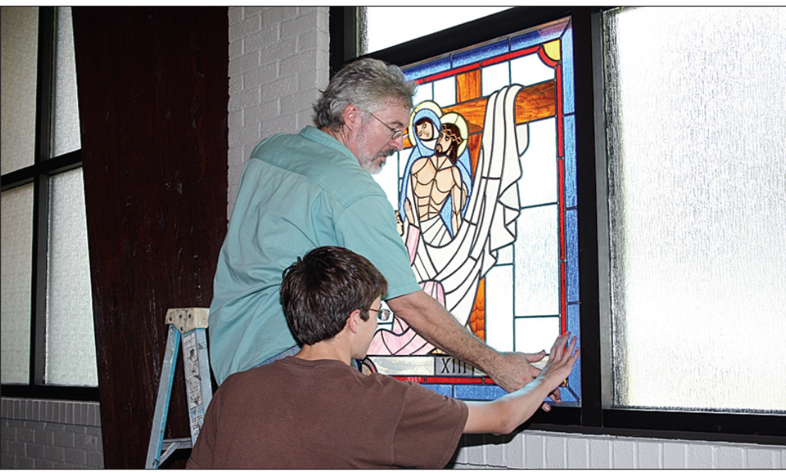
Frank Thompson, left, and his son, Levi, install one of the 14 Stations of the Cross in Our Lady Star of the Sea Church in Cameron. Here they put the finishing touches on the 13th Station - Jesus is taken down from the Cross.
