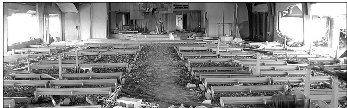
The remains of the kneelers at Sacred Heart of Jesus in Creole provided a solemn commentary on Hurricane Rita not long after people were allowed back into Cameron Parish.
