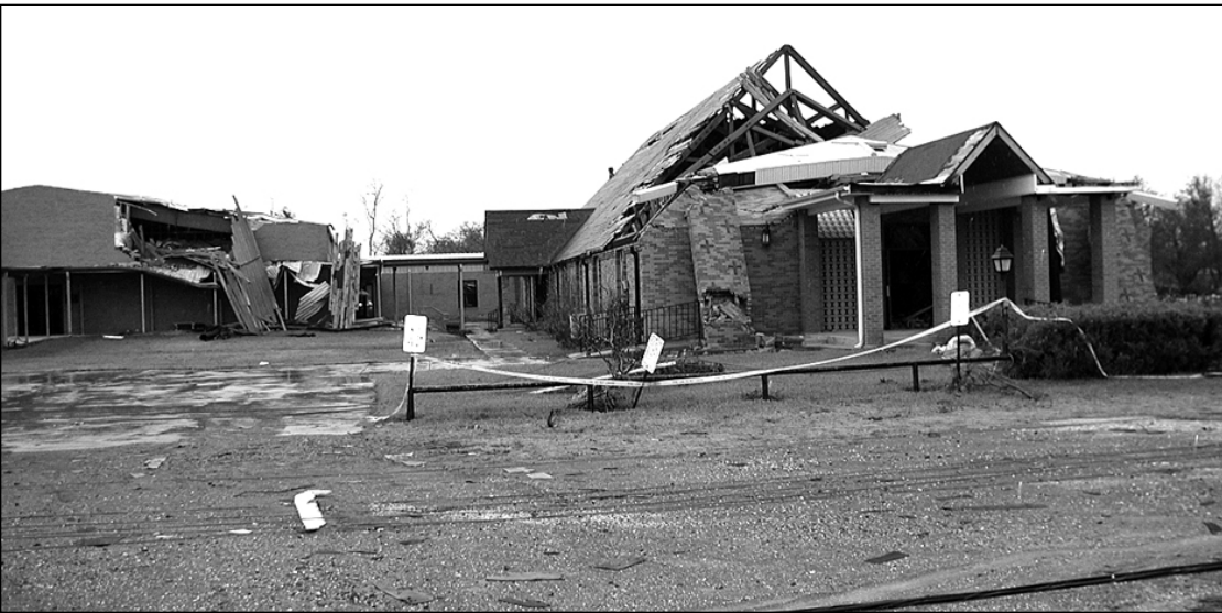
The damage done to St. Peter the Apostle Church in Hackberry is seen some two weeks following Hurricane Rita. The parish is still celebrating Mass in the damaged parish hall. Work has begun in earnest at St. Peter in its rebuilding efforts. Repairs to the religious education building and parish hall await completion of the church.
