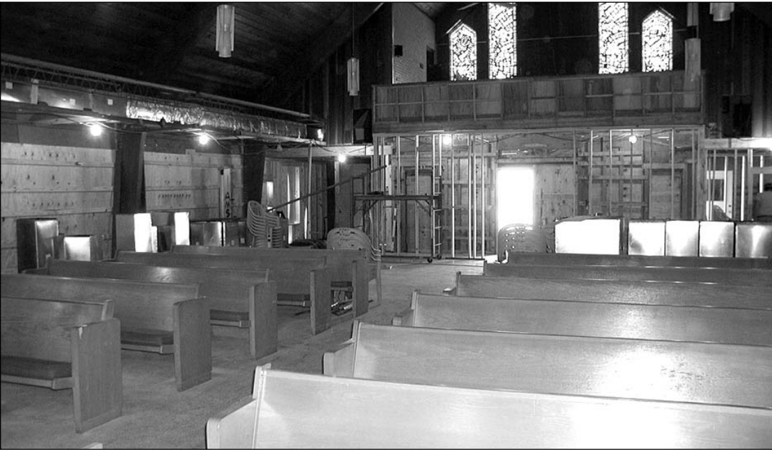
Work has begun on the church at St. Eugene. Much work remains inside and outside before the church can safely be used to celebrate Liturgy.
