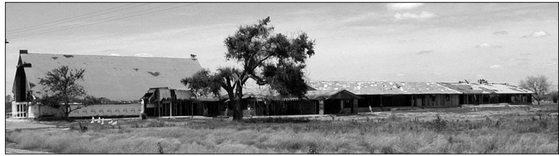
The entire physical plant of Sacred Heart was damaged. Here the church, rectory, hall and religious education building can be seen. The sides of the church were blown out by the surge of the water, which also devastated the rectory, hall and religious education building. Plans continue to be made on the reconstruction of the church.
