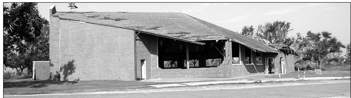
The outside of Our Lady Star of the Sea remains as it was following Hurricane Rita's passage. Debris from the remains of the church's rectory, religious education building and parish hall have long been cleared away.
